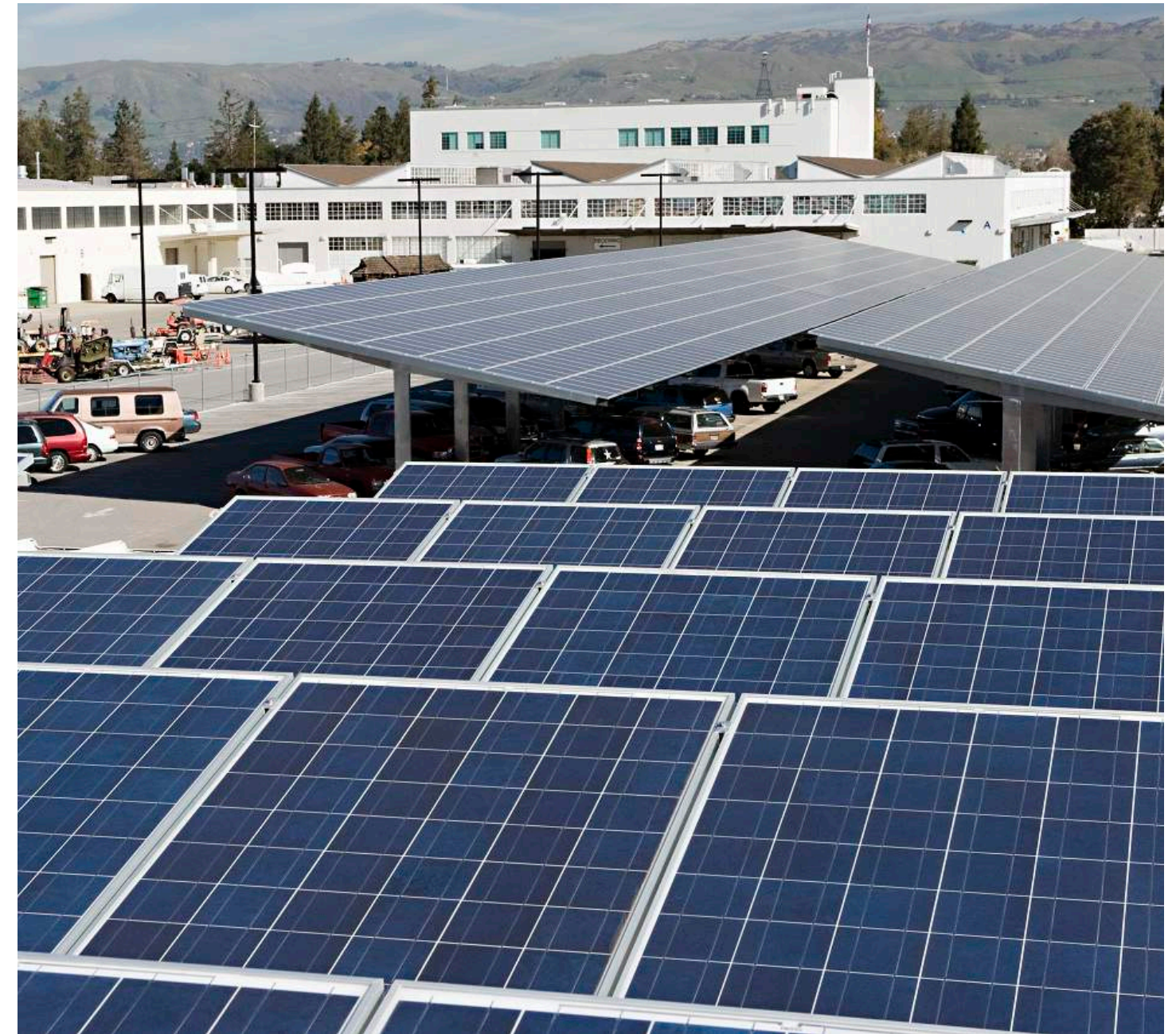
Solar Canopy Parking Lot (San Jose, California)
